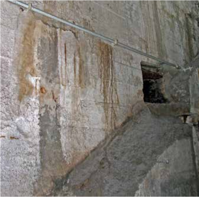
Traces of an intended escalator for passengers to transfer between lines. Photo Jonny B Kirchhain
